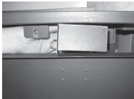
DC Spark Box Bracket Assembly partially removed.
