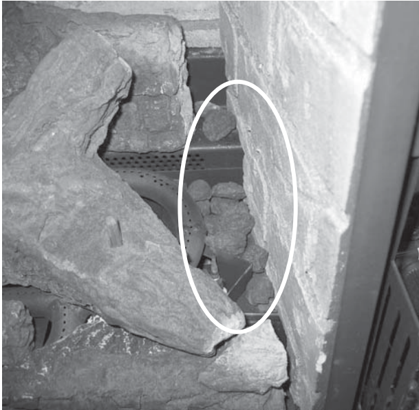
Right side of Burner
