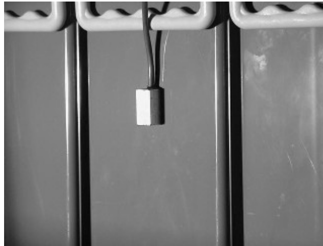
Figure 3.8-3 Typical location of Battery Temperature Probe
