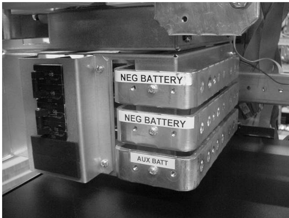
Figure 3.8-1 Battery Cable Connections
